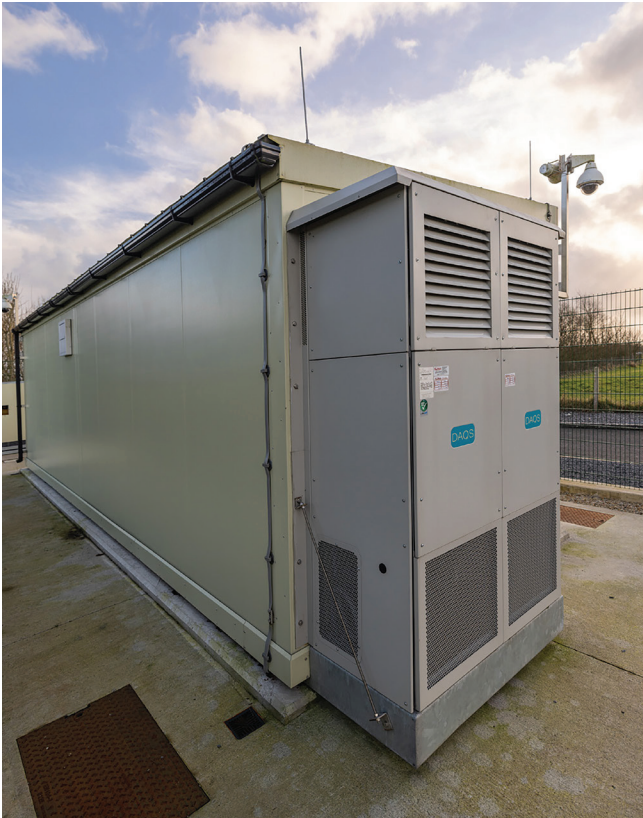
Figure 6. Air conditioning Unit
