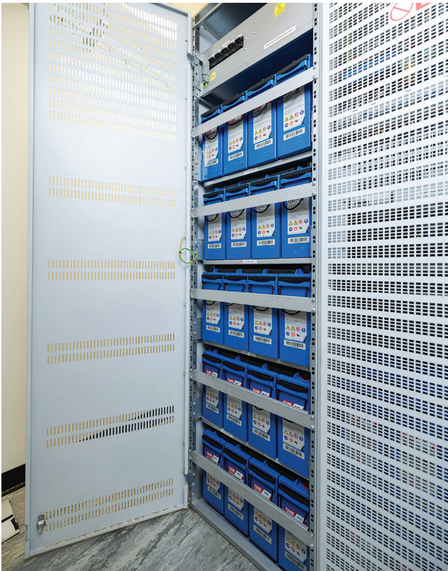
Figure 4. Typical rectifier and battery cell set up
