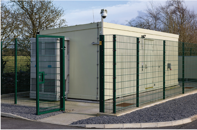
Figure 1. Gaybrook co-location facility
