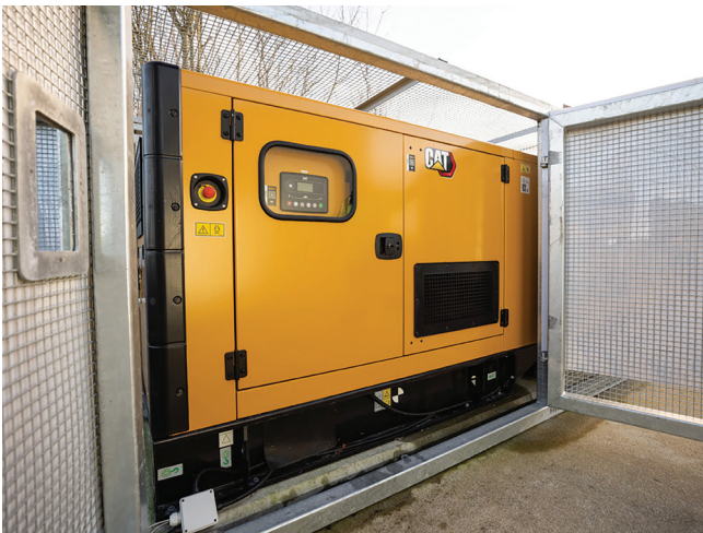
Figure 3. Diesel backup generator
